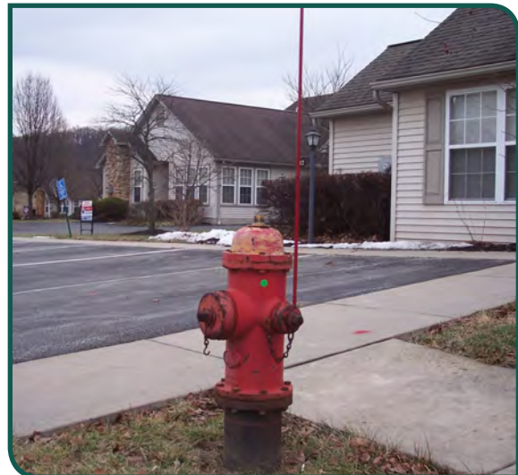
Fire hydrant in Fairfield Borough
