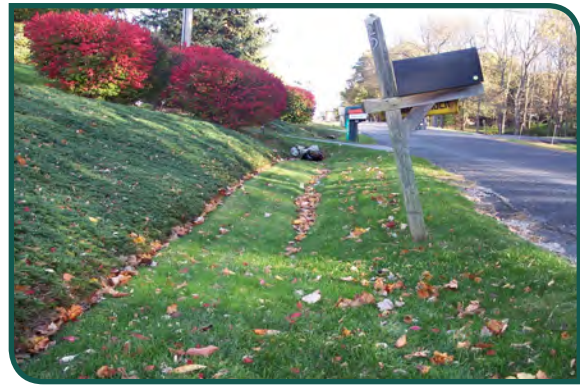
Drainage swales, residential neighborhood, Carroll Valley Borough
